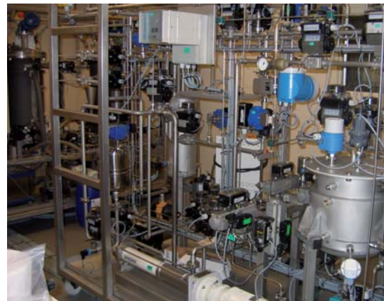
Industrial pilot installation for high standard purification of waste water using membranes
